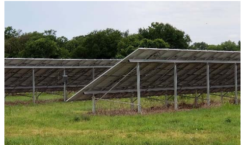
Example of a Solar Conversion System, Ground-mounted
